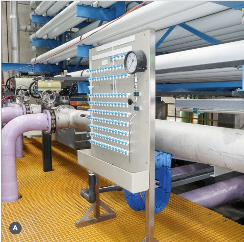
A Overview: Sampling station showing all outlets, complete panel and steel frame. Installed on site.
