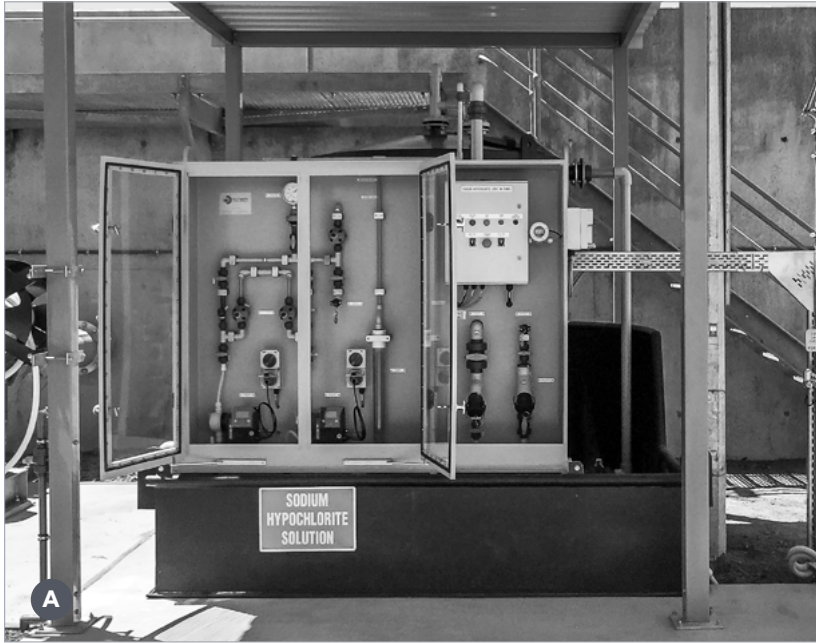
A Front shot: Complete dosing system containing built-in custom fabricated chemical dosing / loading panel, chemical storage tank and bund. The dosing panel is situated within the tank's bund.
