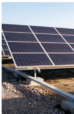
PV array wiring conductor, Spain
