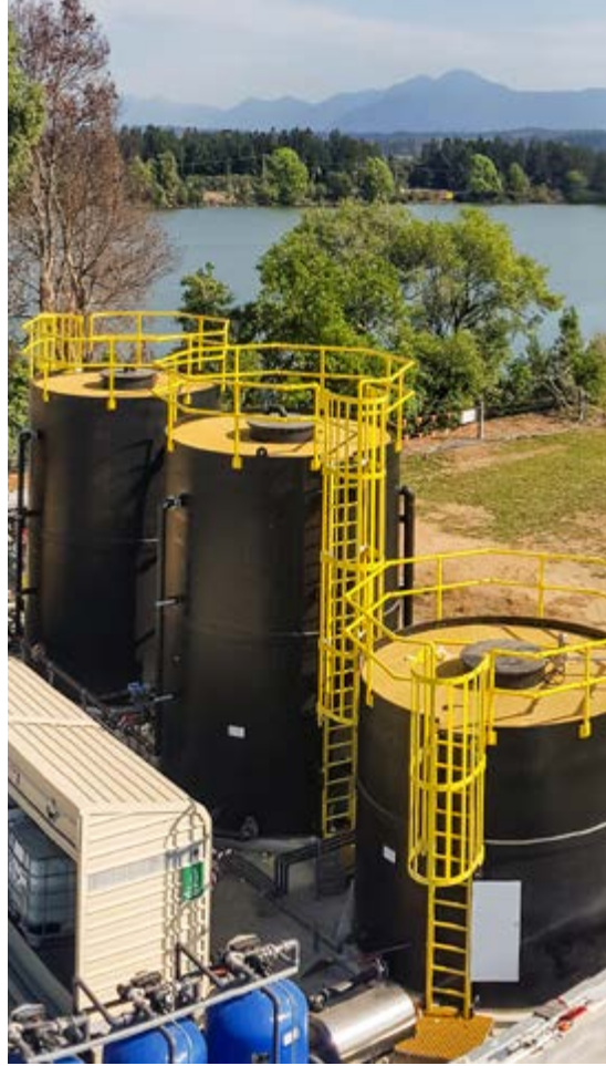
The Fusion PE tanks with FRP top access platforms successfully commissioned at site.
