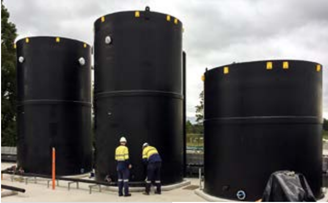
Fusion staff at site assisting with the installation of the wastewater tanks.
