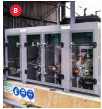
B Fusion designed a cabinet to house the panel and sectioned each system via an internal partition.
