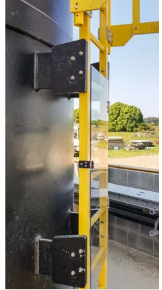
The FRP ladder affixed to the side of the PE tank.
