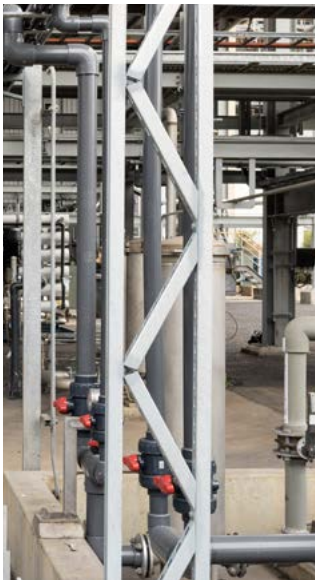
Pipework coming down from the overhead cable trays.
