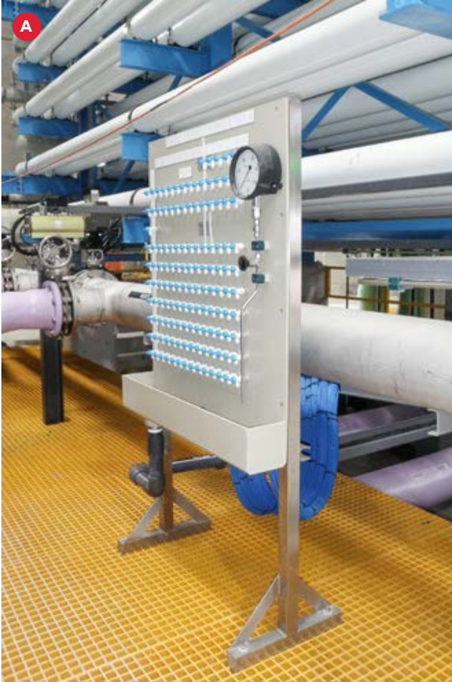
A Sampling station showing all outlets, complete panel and steel frame. Installed on site.
