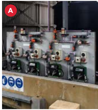
A This existing panel required screening but with the option to isolate the pumps separately and still be able to safely maintain the system.
