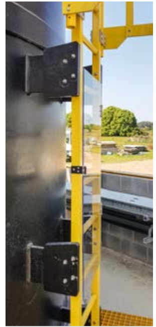
Close up of the FRP ladder affixed to the side of the PE tank.
