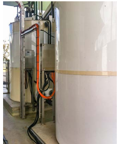
Right: Photo of the existing tanks on site which the client requested be replaced.
